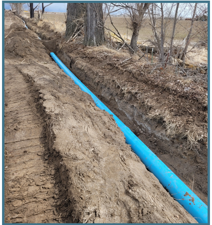
18" PVC pipe delivers water to water users while ensuring that water loss is minimal
