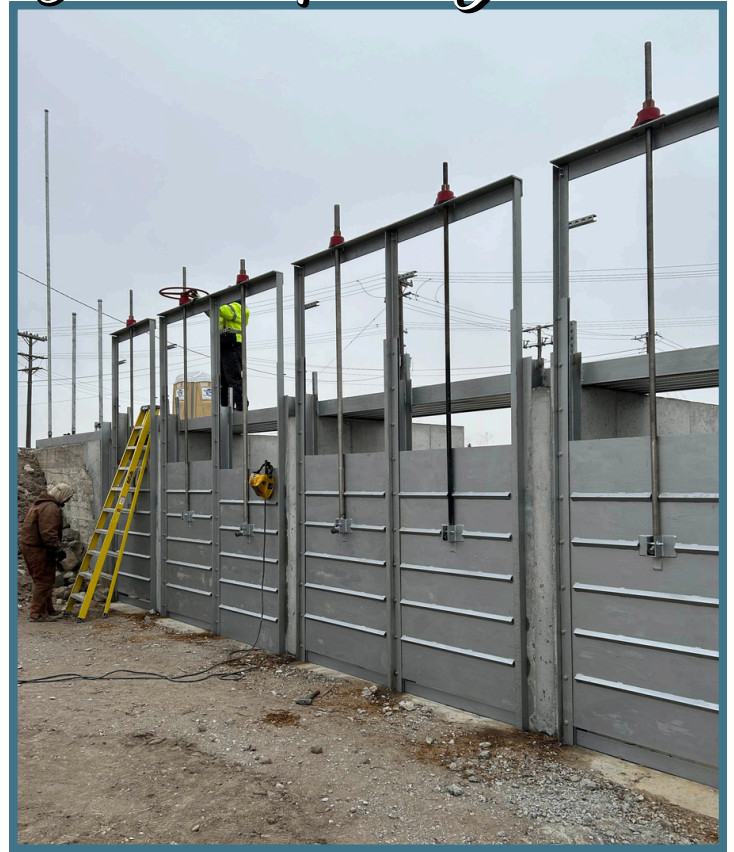
The new gates at the B2 Check Structure. The gates are 6' tall
